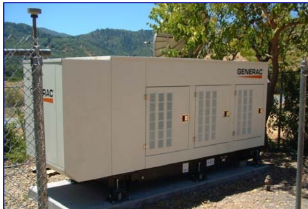
Back Up Generator
